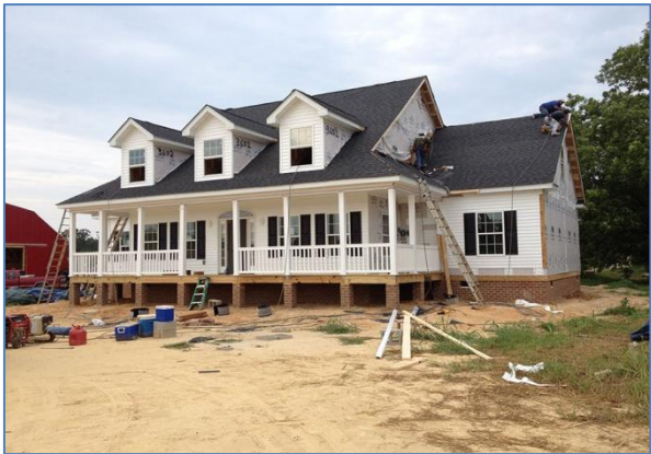
Modular Home (Under Construction) Individual modules delivered to the site and assembled on a permanent foundation
